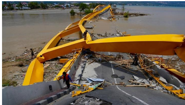
Figure 5. Destroyed Bridge in Palu After September 2018 Tsunami Isolated Palu City From Aid (Source: Aljazeera 2018)
